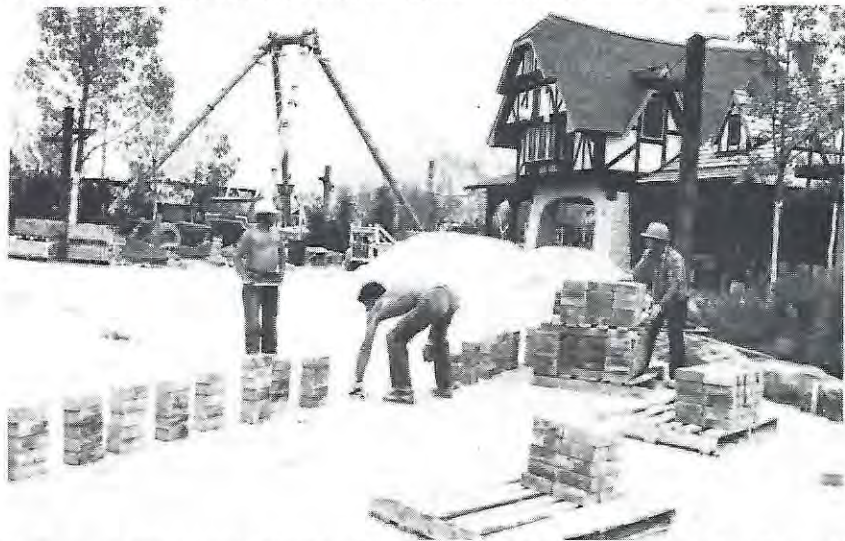
Workers laying some of the 2,900,000 cement pavers used in the park's walking areas. Note viking ship in background.
