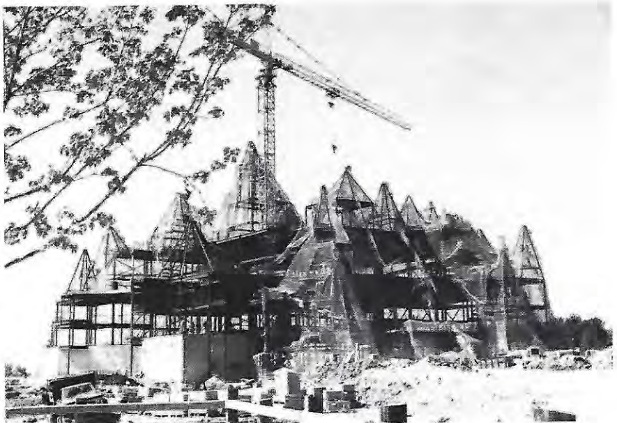
The mountain, prior to the spraying of concrete. Note the wire mesh used for forming the mountain-like appearance.
